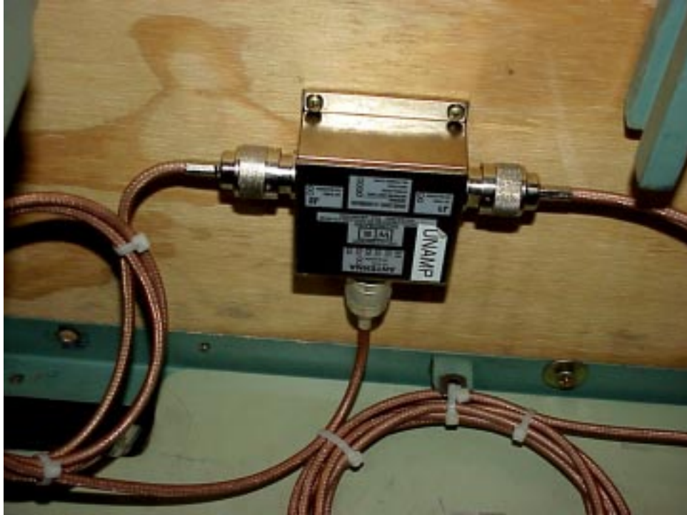
Figure 19. HC-130 GPS splitter mounted below radio table
